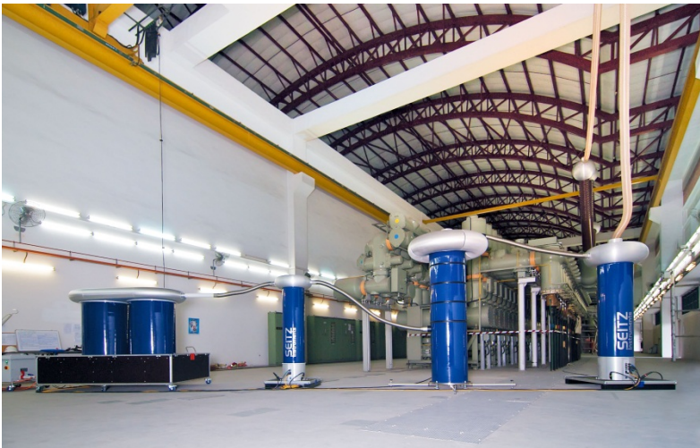
onsite high voltage products in operation
